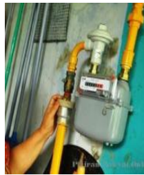
Gas from public system
